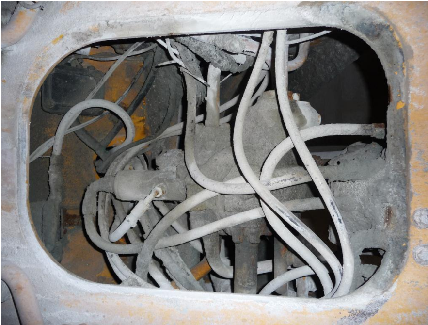
Figure 5: front hydraulic compartment untreated after 6 years
